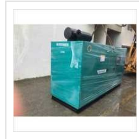
15 KVA Pre Owned Cummins Diesel
